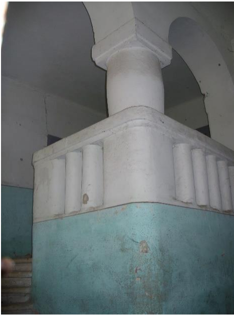
Figure 10 Evangelical School in Bruiau, detail of the staircase, picture taken by the author, 2016.
