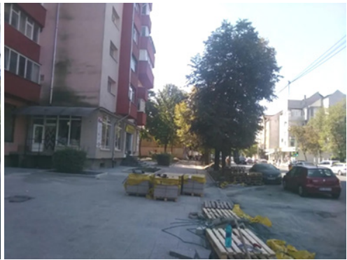
Fig. 3. Pedestrian alley landscaping, decking, and cladding; Street improvement, decking and cladding (own source)
