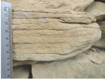
Fig. 2. Severe delamination along the bedding planes.
