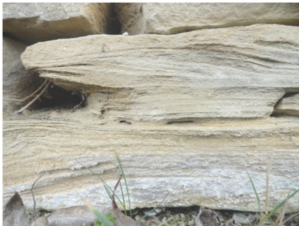
Fig. 4. Delamination and granular disintegration.
