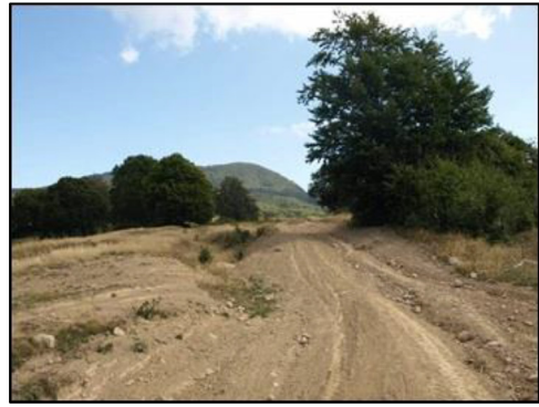
Fig. 2b. Linear erosion processes on forest roads
