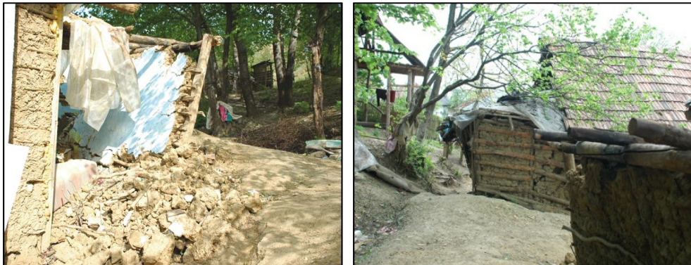
Fig. 4. Adobe houses damaged by the Chelița landslide
