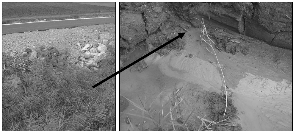
Fig. 6. Former mud pool, filled with rocks (left) Reactivated mud volcano (right) Mihăileni, Harghita county.
