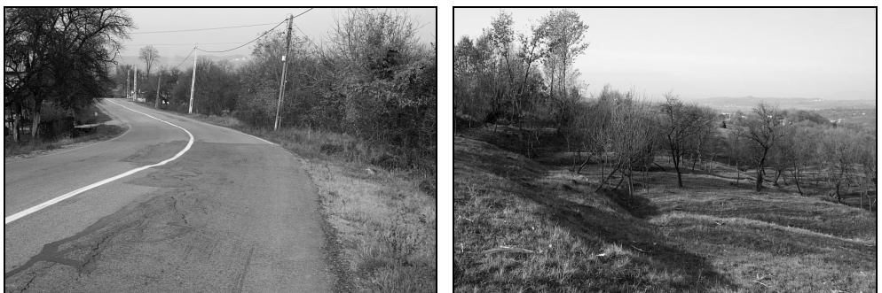
Fig. 10. The road DN 18B from Baia Mare to Tg. Lăpuș (left) and recent landslide movement indicated by tilted young trees in Cărbunari area (2012).
