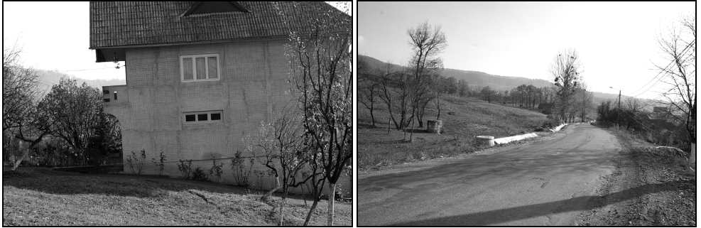
Fig. 8. Active failure near house indicated by cracks and tilted young trees (left) and the DJ 184 road in Baia Sprie - Șișești area (2012).
