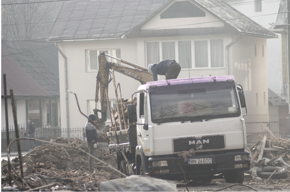
Fig. 8. – The demolition of the Dr. Ciuta Sanatorium in the summer of 2018, after years of disputes regarding its ownership. Source: author.
