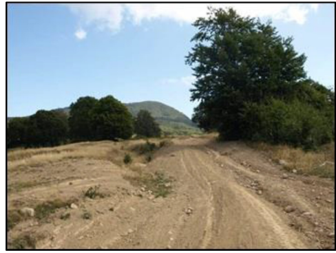
Fig. 2b. Linear erosion processes on forest roads
