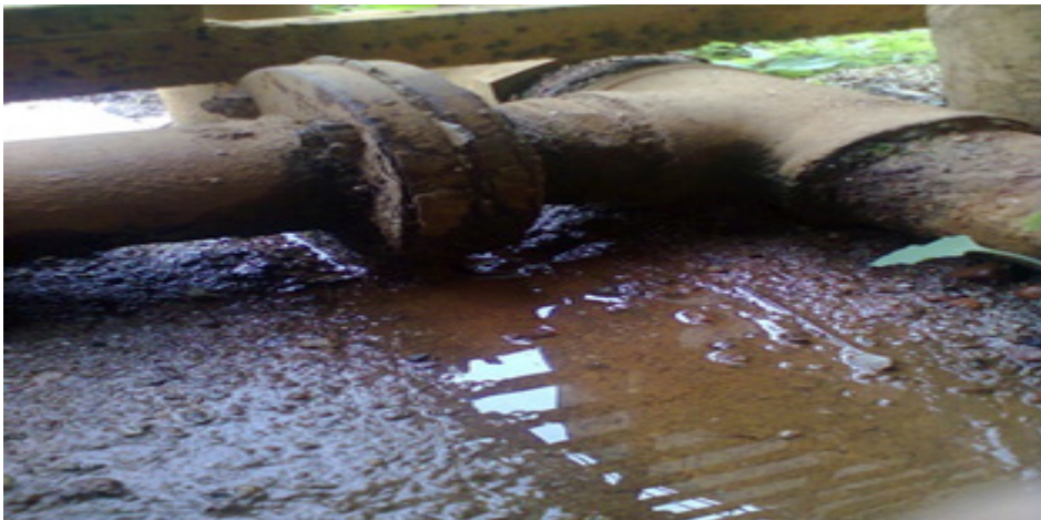
Figure 2. Leakage from the burst pipeline
