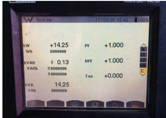
Figure 5. Measured power and power factor values for the photovoltaic installation
