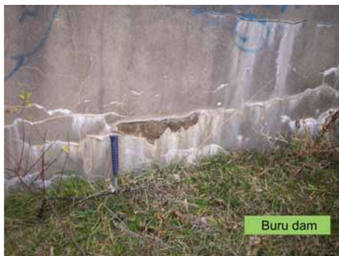
Figure 1. Fissures with carbonate deposits at the base of Buru dam (Cluj County).
