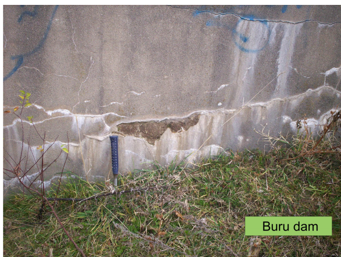
Figure 1. Fissures with carbonate deposits at the base of Buru dam (Cluj County).
