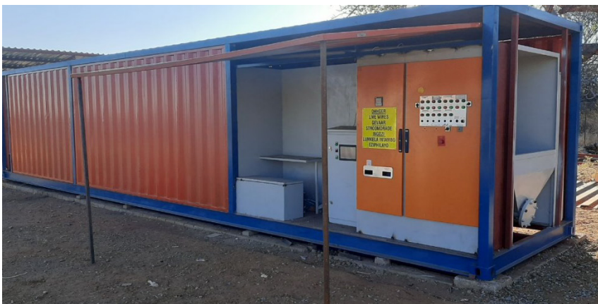
Figure 8. Electrical and control system panel
