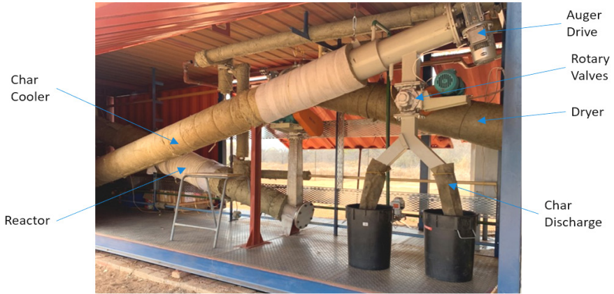
Figure 6. Main process equipment
